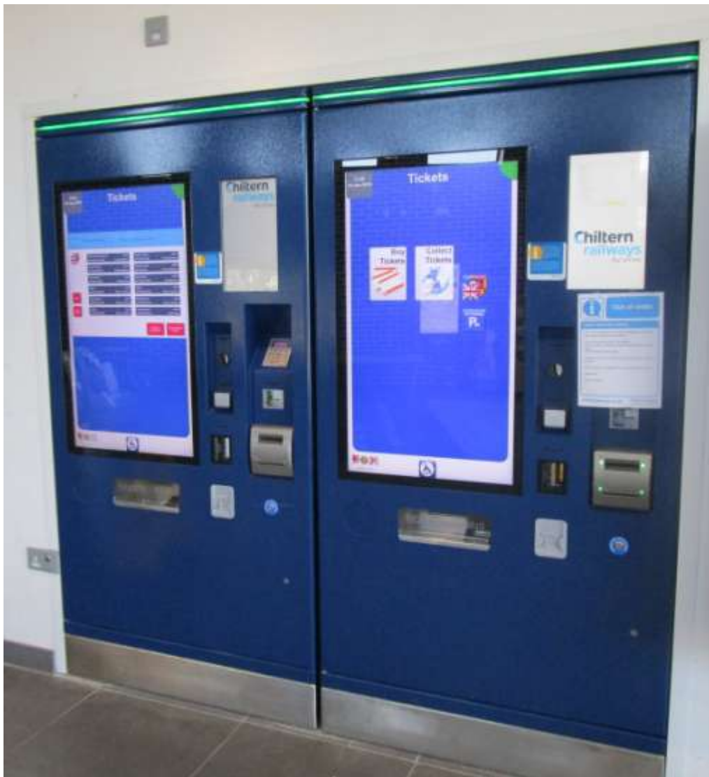
Two TVMs installed inside the main entrance at Bicester Village station
